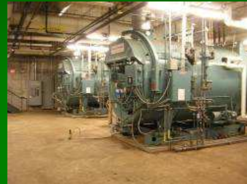
Steam Plant Decentralization & LP Conversion
