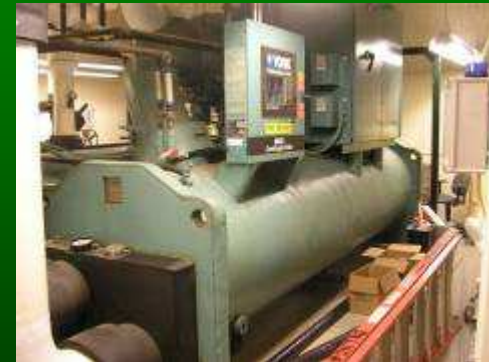
Variable Speed Chillers
